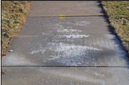
Excessive salt on the sidewalk
